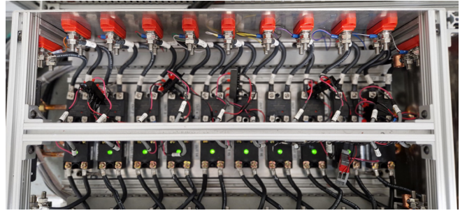
FIGURE 3. Chiller Plate with Mounted SSRs
